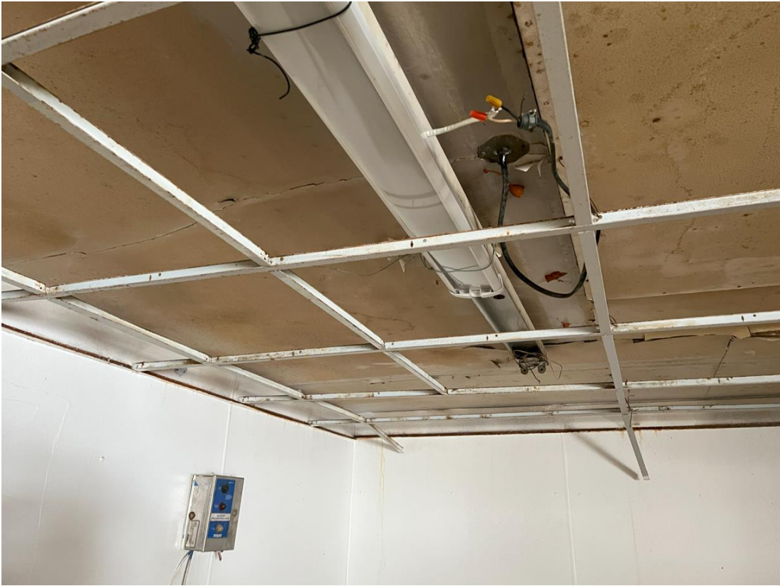
Photo 19 – Damaged electrical lighting in the kitchen
