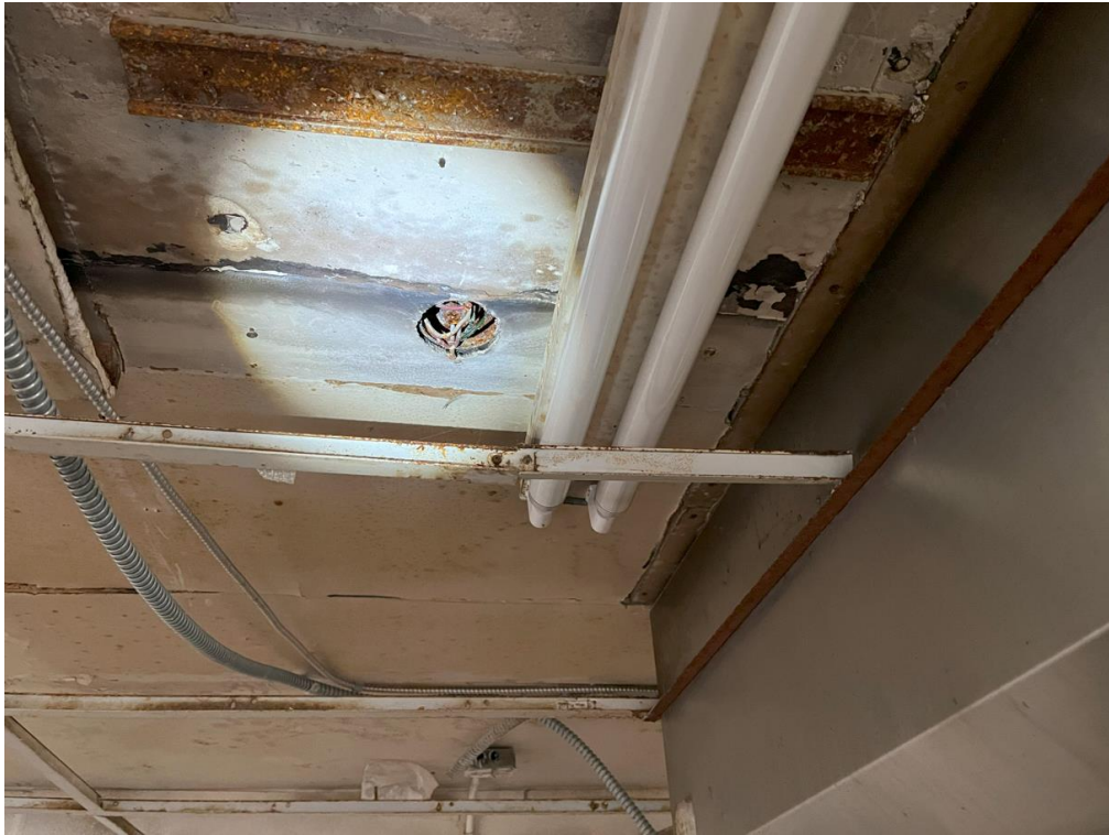
Photo 21 – Questionable electrical wiring in the kitchen
