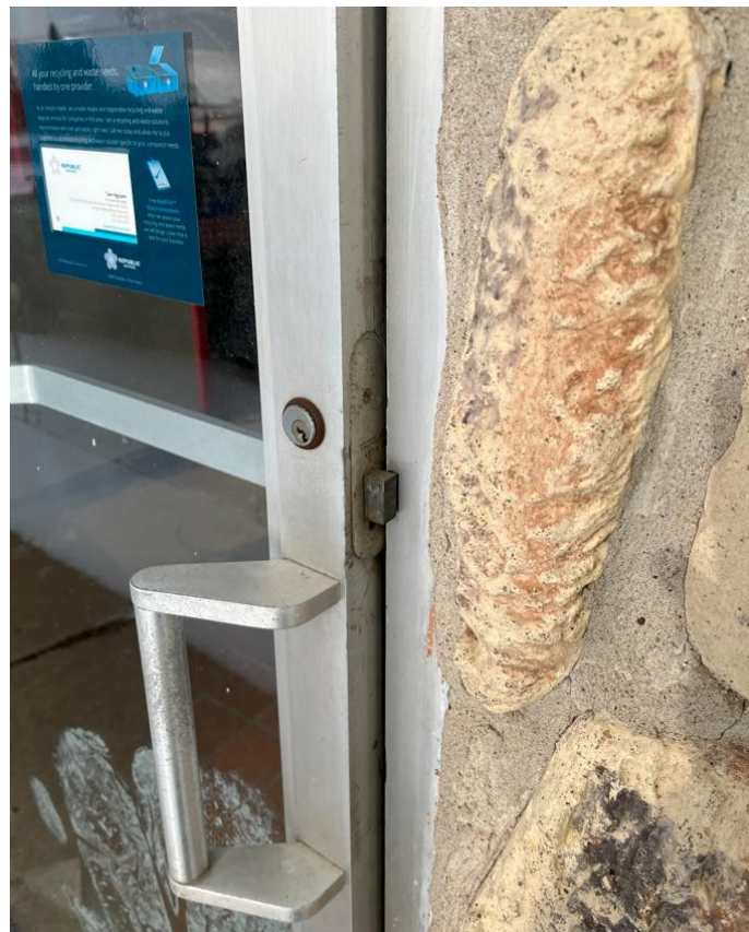
Photo 2 – Photo of the front entrance propped open by the dead bolt
