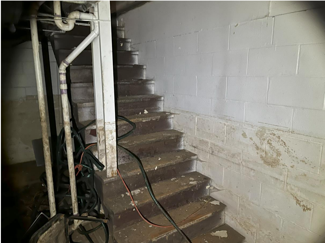
Photo 40 - Appears that the basement has filled with water to approximately 4 feet
