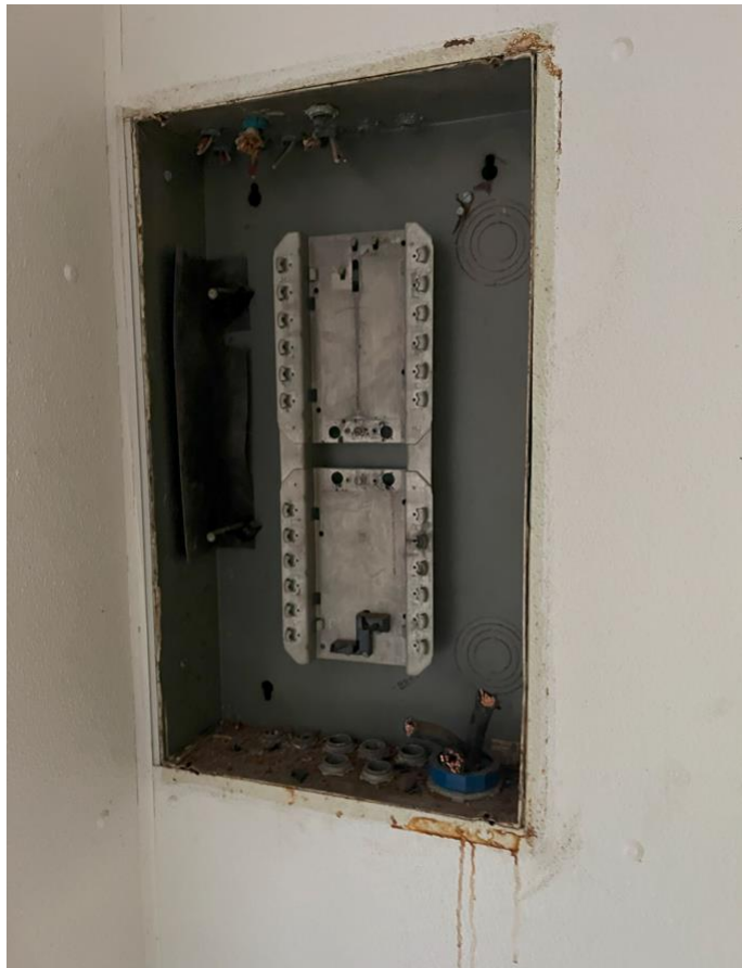
Photo 22 -Electrical panel in kitchen has been stripped of all breakers and wiring
