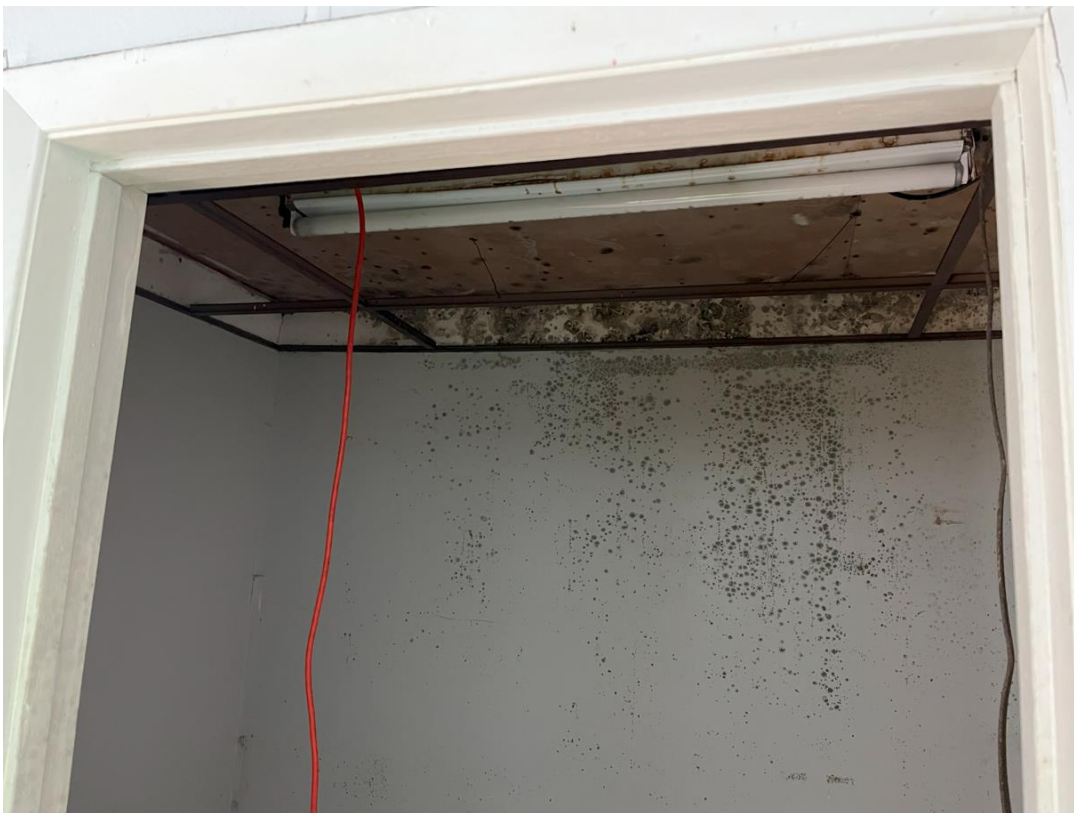
Photo 24 – Signs of roof leaks and mold growth
