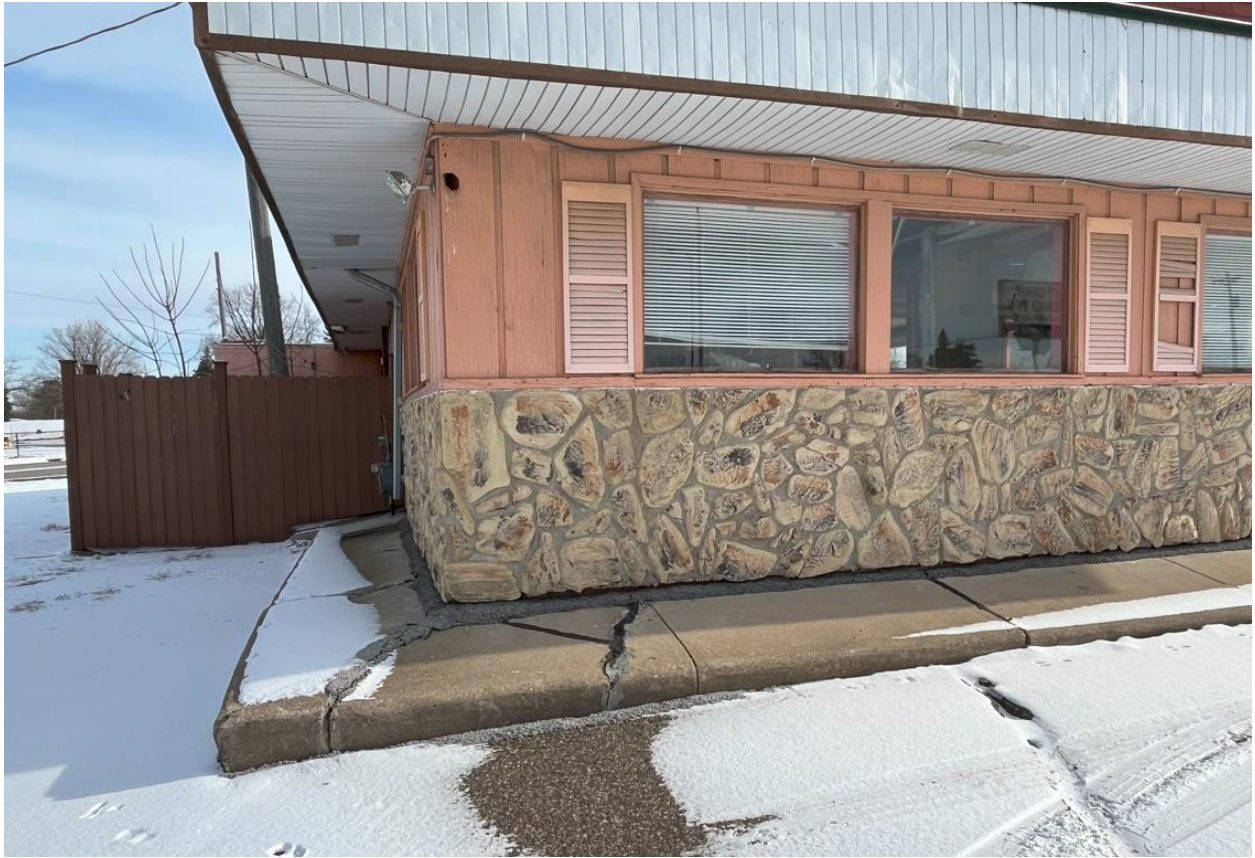
Photo 29 – Back corner of the building with cracked and settling sidewalks
