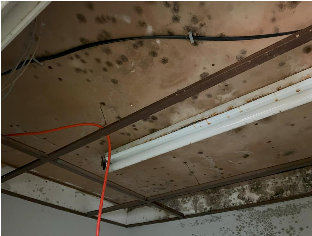
Photo 25 – Additional signs of moisture and mold growth in the kitchen office
