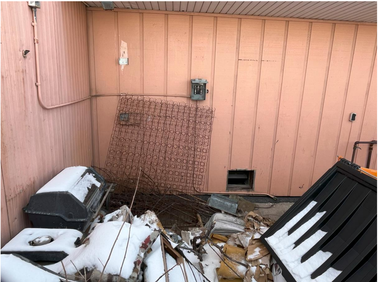
Photo 33 – Rubbish and debris in the fenced area at the back of the building
