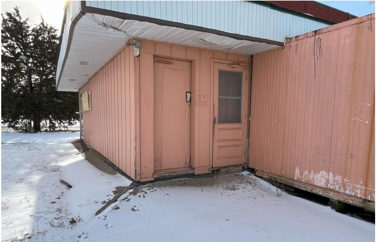
Photo 35 – The foundation for the exterior walk-in cooler at the rear of the building was failing such that the cooler was pulling away from the exterior wall.
