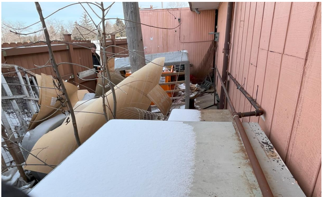
Photo 34 – Rubbish and debris in the fenced area at the back of the building
