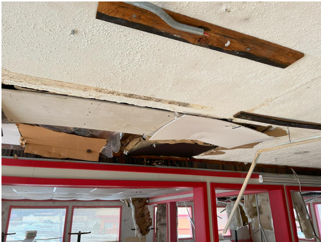
Photo 13 – Ceiling above the front entrance with patches in the ceiling
