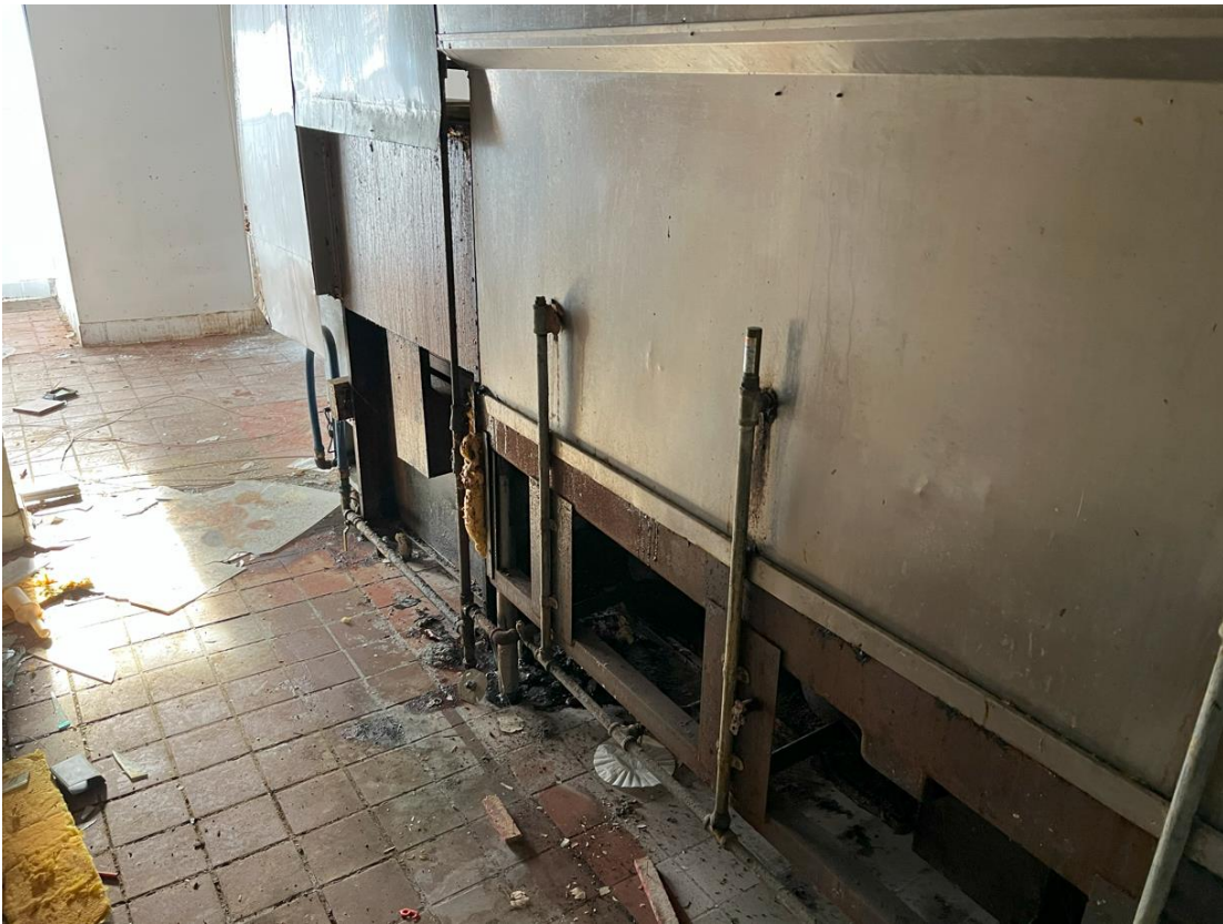
Photo 17 – Back side of the cooking line and hood
