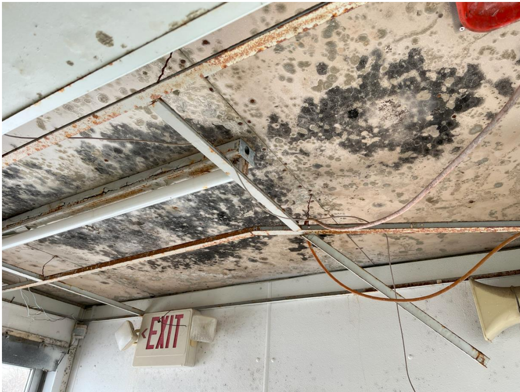
Photo 23 – Signs of roof leaks and extensive mold growth
