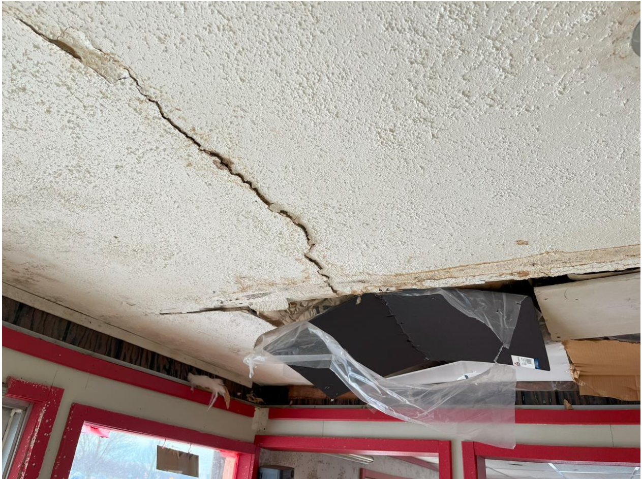
Photo 14 – Photo of the condition of the sheetrock ceiling
