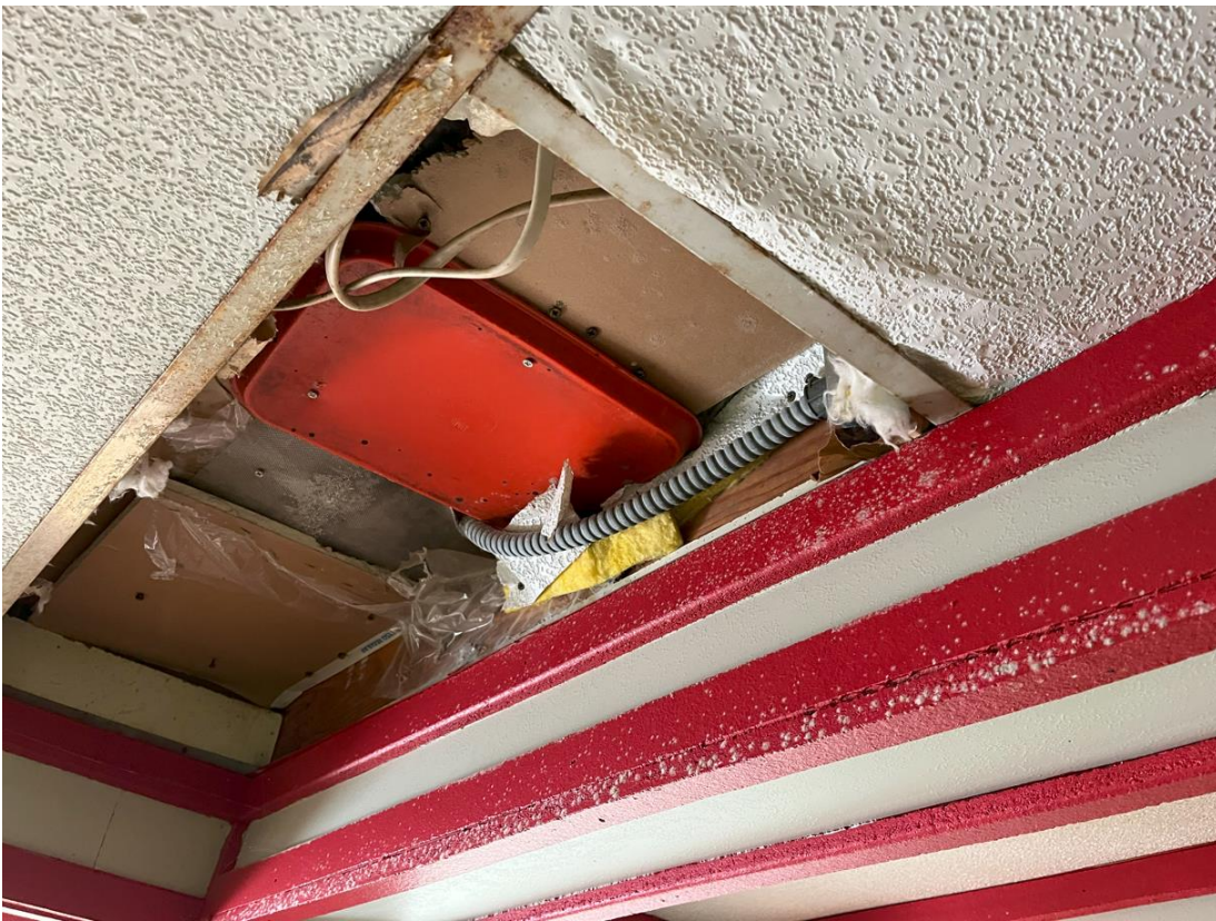
Photo 11 -Ceiling with plastic tray blocking holes in the ceiling
