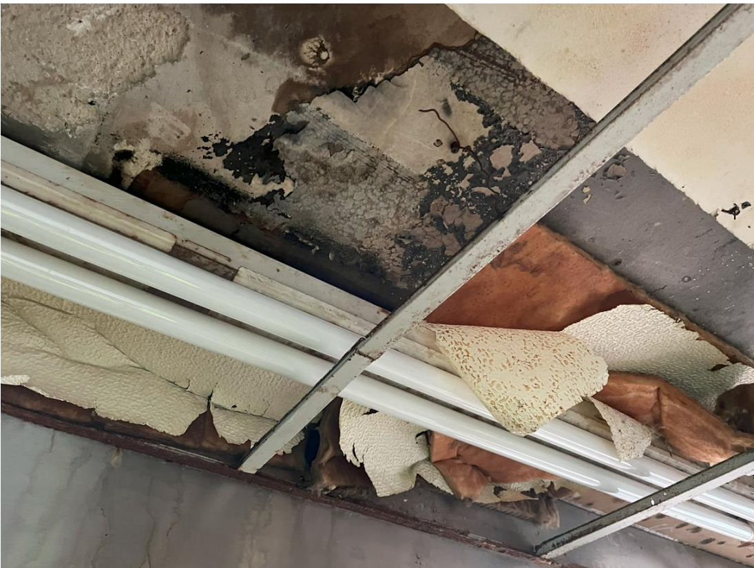
Photo 20 – Deteriorated ceiling area in the kitchen
