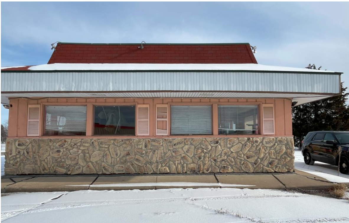
Photo 28 – Sidewalks around the building settling
