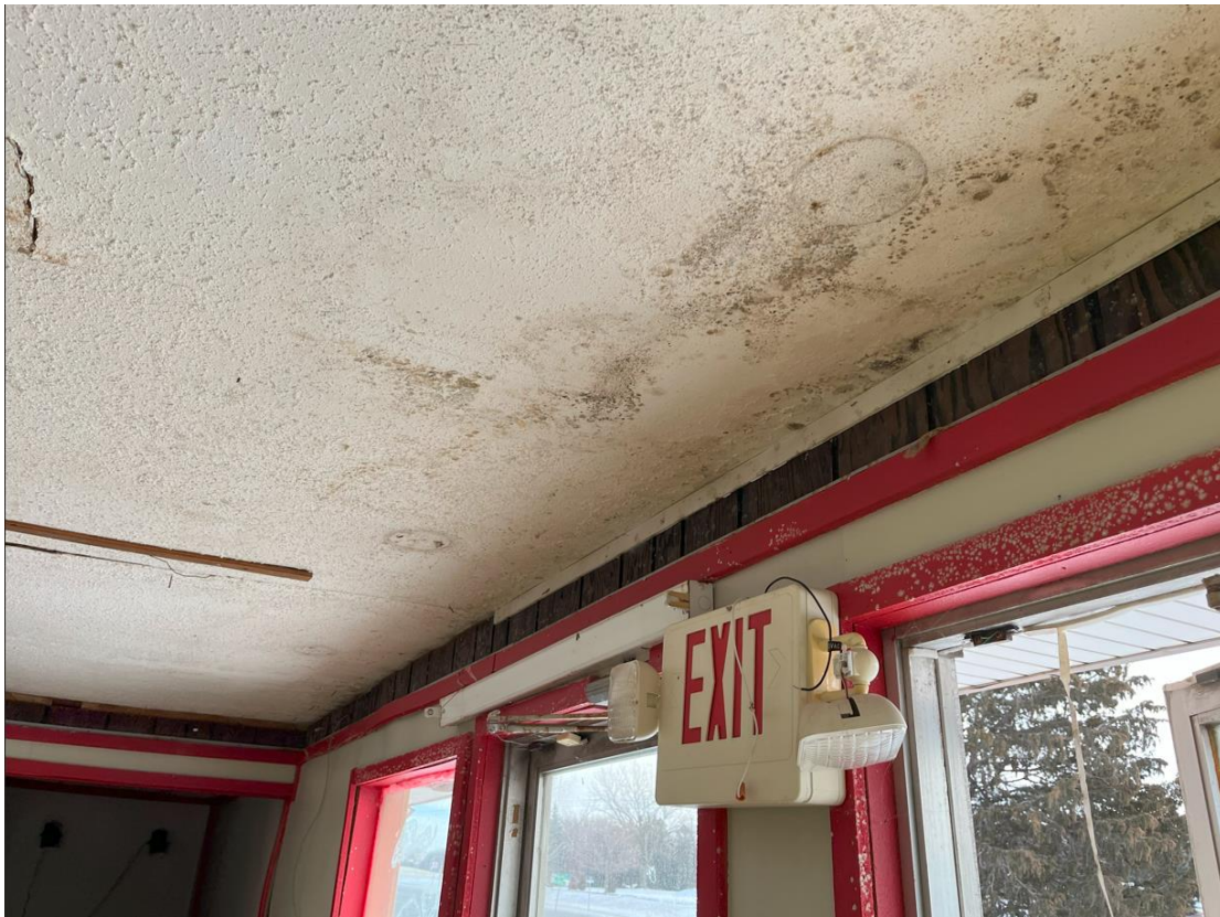
Photo 8 - Photo showing what appears to be mold on ceiling
