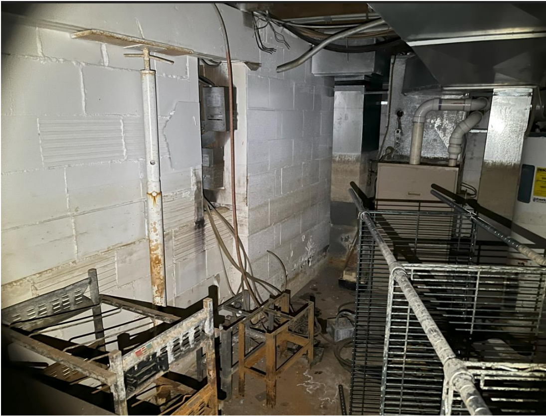
Photo 38 – Rubbish in the basement
