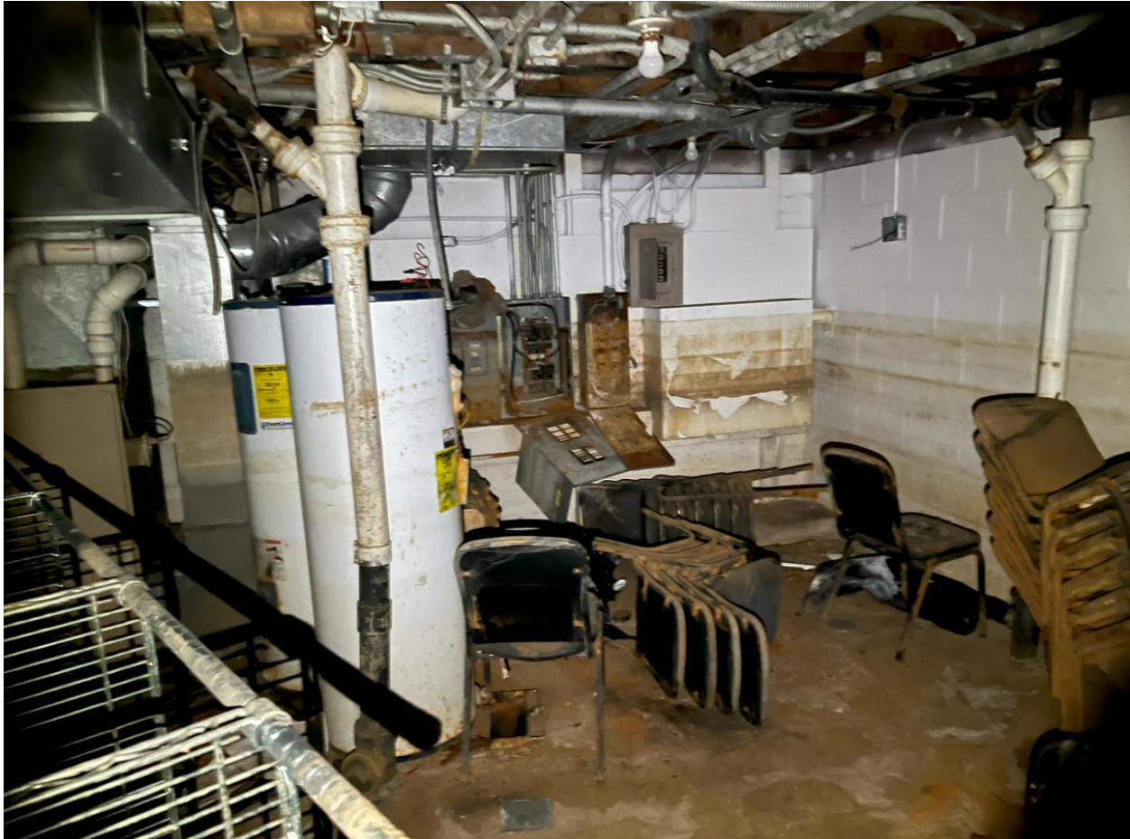
Photo 37 – Basement showing water damage and signs of being flooded
